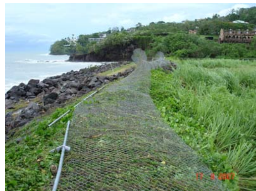
Photo 7 – Damage to Fence at GFL Charles Airport
