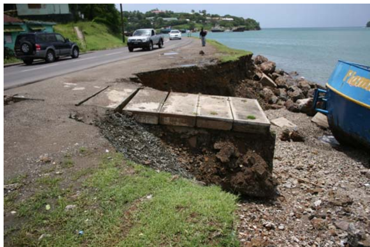
Photo 2 – Damaged culvert and slope protection
