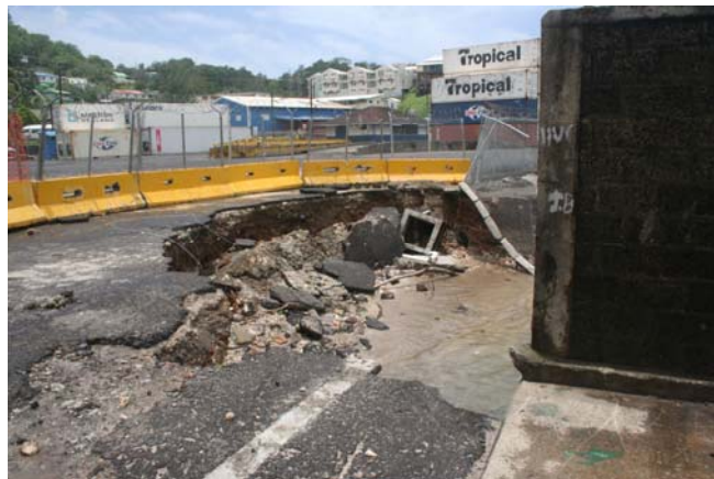
Photo 5 – Damage to section of pavement at Shed 7
