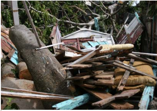
Photo 1 – Completely destroyed house at Gros Islet
