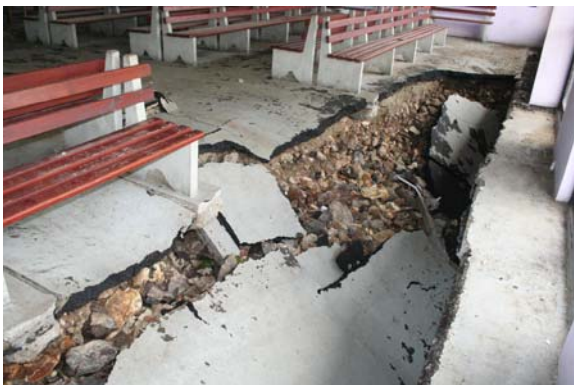
Photo 6 – Damage to section of Ferry Terminal
