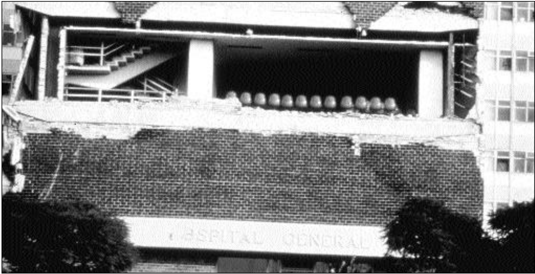
Photograph 17. The addition of aesthetic features on buildings can increase their vulnerability in earthquakes.
