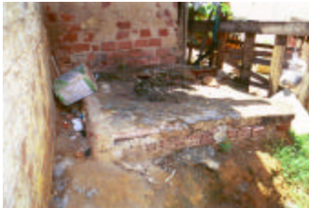
Abandoned and/or unimproved pit latrines are ideal breeding sites for Culex quinquefasciatus , and should be filled up with dirt and replaced with VIP latrines or sanitary sewerage. Photo by Steven Ault, 2003.
