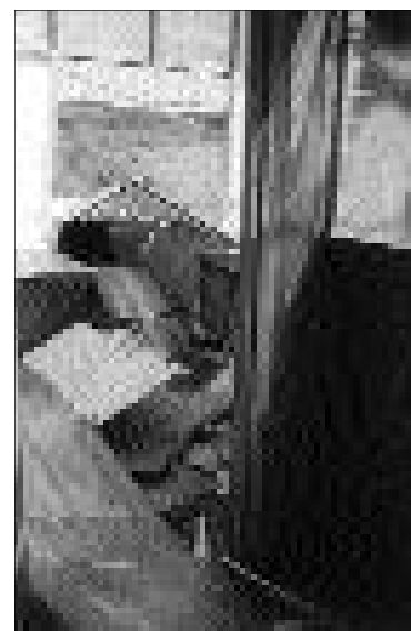
During Hurricane Luis the roof, windows, doors, power and water supply were all lost in the building that housed the Antigua Emergency Operations Center and offices of the Ministry of Health, pictured here.
