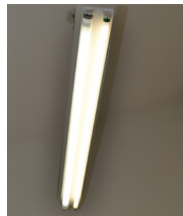
Fixture with a 32 W and a 40 W fluorescent lamps in operation at MION Source: PHS. Lighting Audit Report
